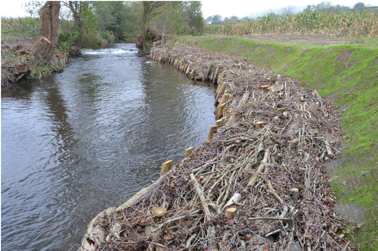
Figure 3.1. Newly installed revetments comprised of willow and brush designed to provide a living barrier and protect against future bank erosion along the Afon Cain, Llanfechain, 2018.
